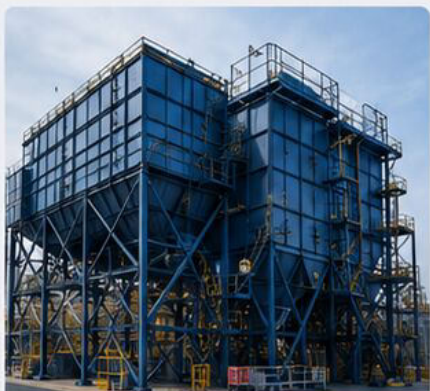
BAG HOUSE SYSTEMS
